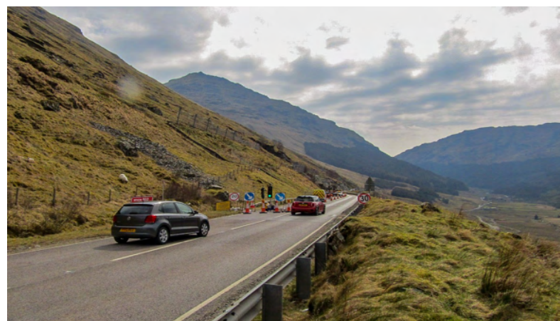
Top left: Aerial view of the August landslips. Top right: Teams carry out slope assessments. Above, top: OMR temporary bund completed. Middle: Work continues with additional mitigation measures at the RaBT. Bottom: Traffic lights in operation after replacing the convoy system in April.
