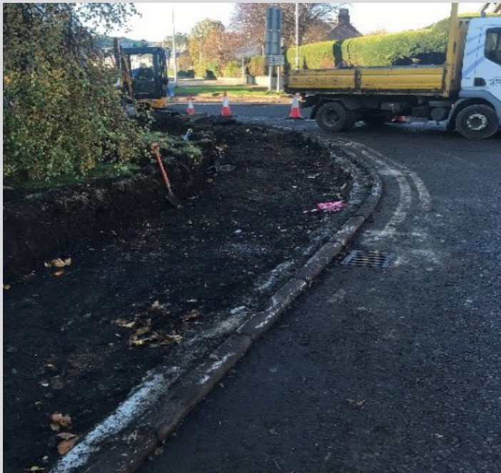
The kerbing works at Montague Row are progressing well. The crossing is expected to be finished in January 2021.
