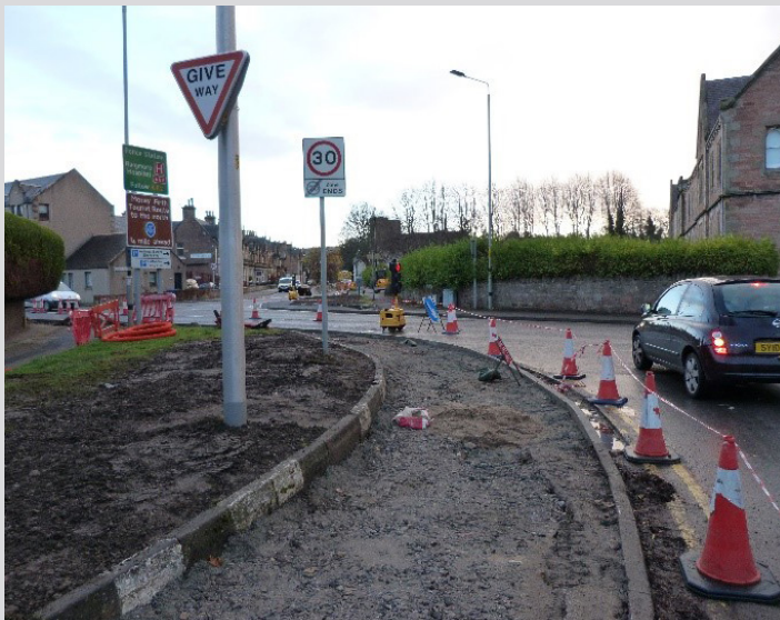
The new footway on Bruce Gardens is expected to be finished in January 2021
