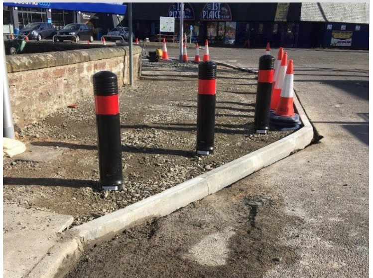
A82 / Smith Avenue Junction: Image showing the kerbed build out at Smith Avenue ready for surfacing.
