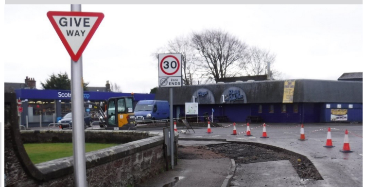
Photo from Smith Avenue to the A82 showing excavation of the area ready for new kerbs.
